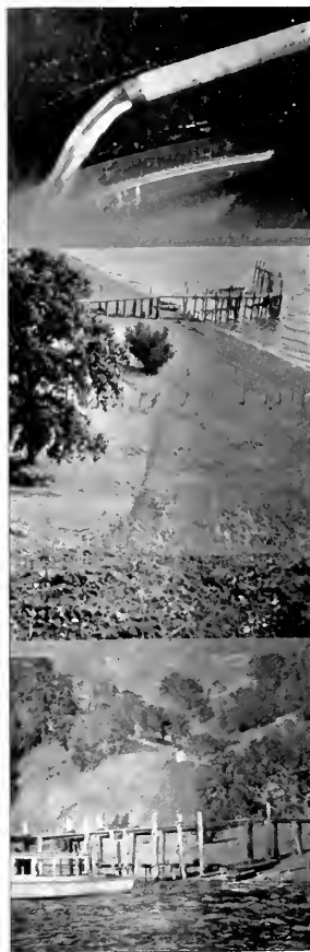
The above three illustrations show the character of the installation of the Sterling gasoline driven pump installed by A. G. Hebben Company of Clear Lake, California. The results of the tests on this installation were described in Pacific Marine Review for July. Note the full steady stream at the tank outlet shown in the upper center.
